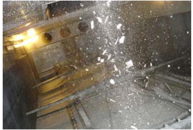
Containerized rake ice storage room
